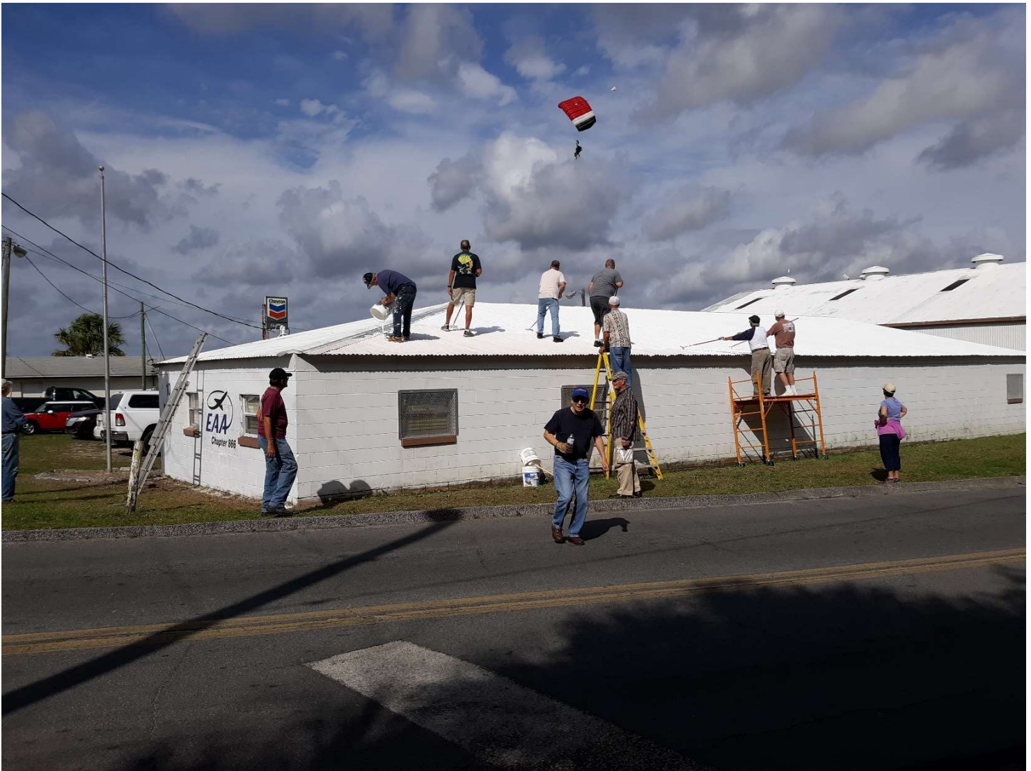
Chapter volunteers work on roof coating project supervised by Bob Rychel Picture by Les Boatright
